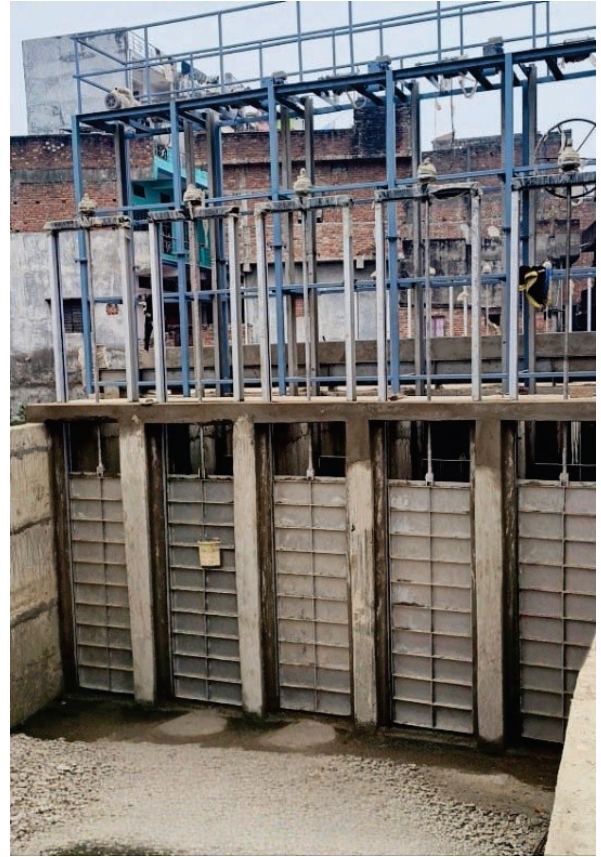
ILLAHIBAGH Pumping Station, Gorakhpur (Gates)
