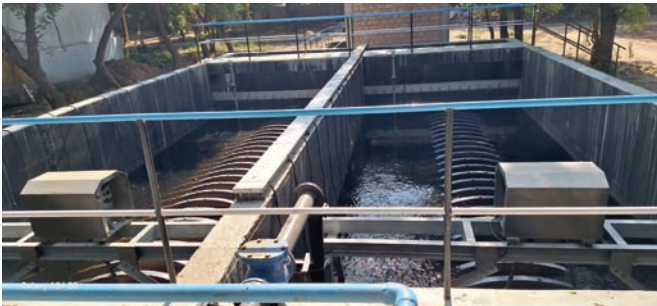
100 MLD STP JODHPUR (Fiber Disc Filter)
