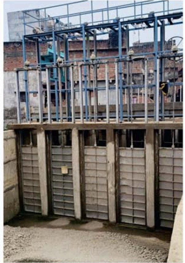
ILLAHIBAGH Pumping Station, Gorakhpur (Gates)
